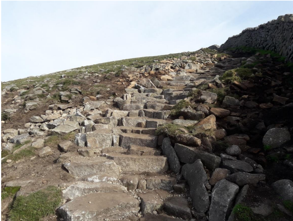
Figure 6.2: The same section of path below the summit of Slieve Donard following reconstruction using stone transported to the work site by helicopter. Image taken September 2021 following construction.
