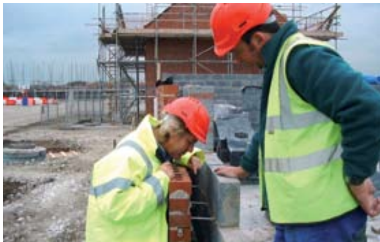
Dr. Roberts from Leeds Metropolitan University and Loftus Construction looking at cavity construction on site
