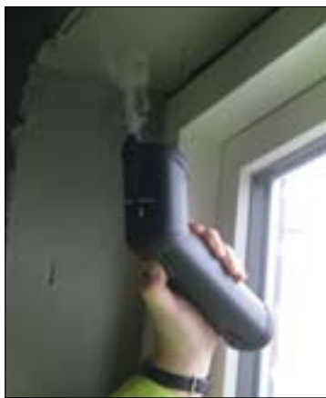
Using a smoke gun to detect air leakages
