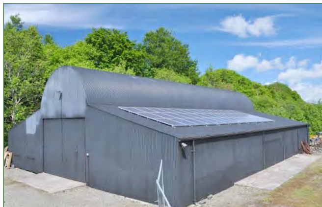
Photovoltaic cells on the roof of the Geler-Jones store at Llanerchaeron. There will be a site visit to see this during the BCAG's Fit For the Future? Conference on 4 April 2012
