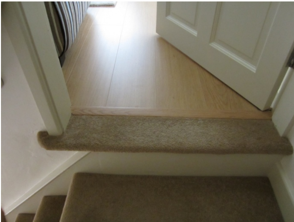
Step at top of stairs into lounge
